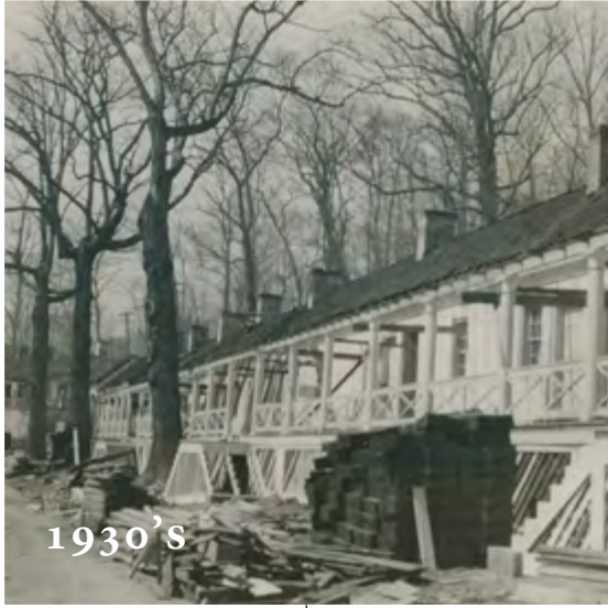
1930's - REPAIRS AND UPDATES TAKING PLACE AT THE PARADISE COTTAGES IN THE 1930'S.
