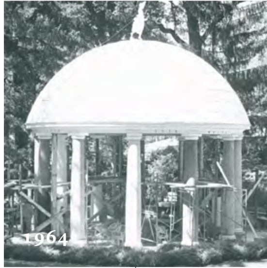
1964 – PAINTERS AND MASONS WORKING DILIGENTLY TO COMPLETE RENOVATIONS OF THE ORIGINAL TWELVE COLUMNS OF THE SPRINGHOUSE.
